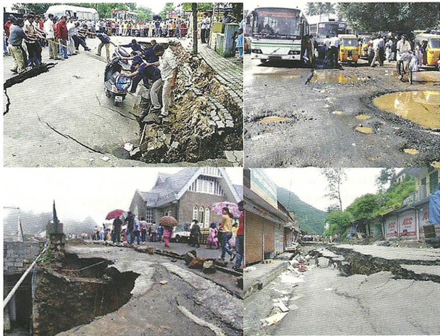
A failed trenchless project would lead to damages to surrounding structures.
